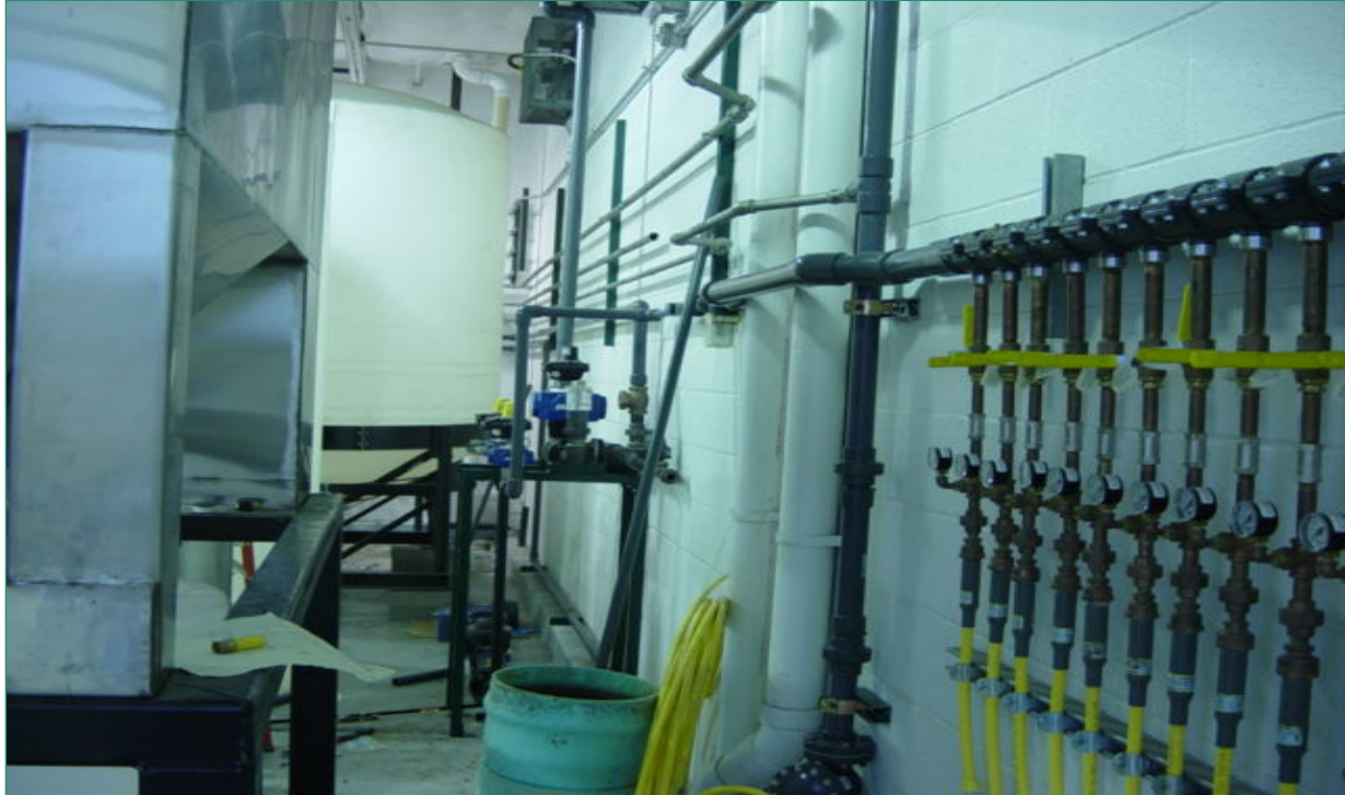
Electron donor storage tank and bioenhancement well network
