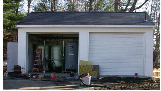
Upgraded system was installed inside newly constructed garage to match site décor.
