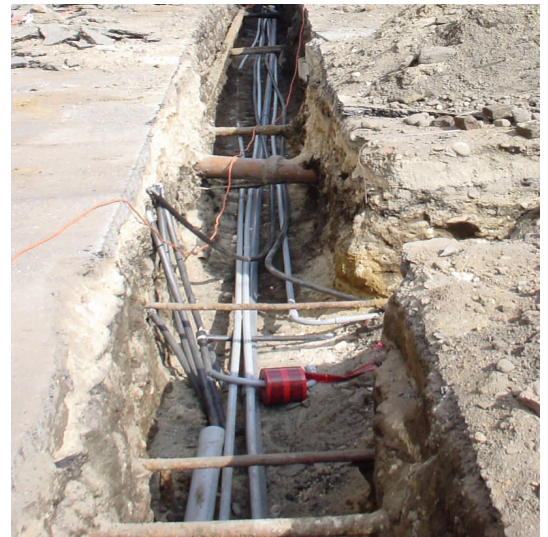
As with many historic industrial sites, subsurface obstructions are numerous. IESI has worked on dozens of MGP sites and is familiar with the nuances they bring.
