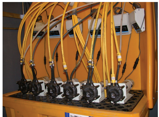
Initial system consisted of timed peristaltic pumps to extract NAPL from bottom of wells
